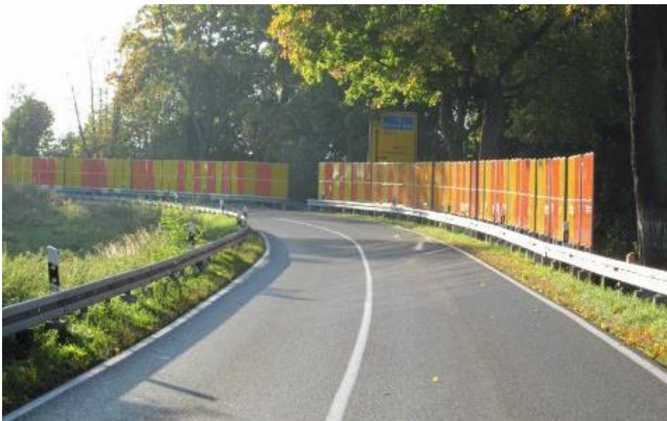
Figure 6.304 - Optical guiding frame in a curve with fatal accidents with integrated optical break (source: Birth, S., Demgensky, B. & Wähler, U., 2016)
