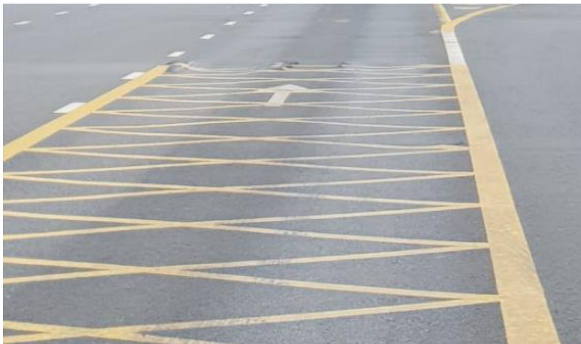
Figure 6.298 - Yellow marks to avoid invasion of heavy vehicles when having traffic jam in the slow lane (increasing of safety from drivers coming from the link road). Detail 3
