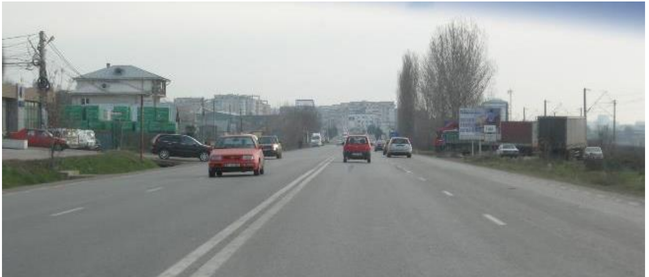
Figure 6.106 – Before the first intervention: lanes without newjersey separation
