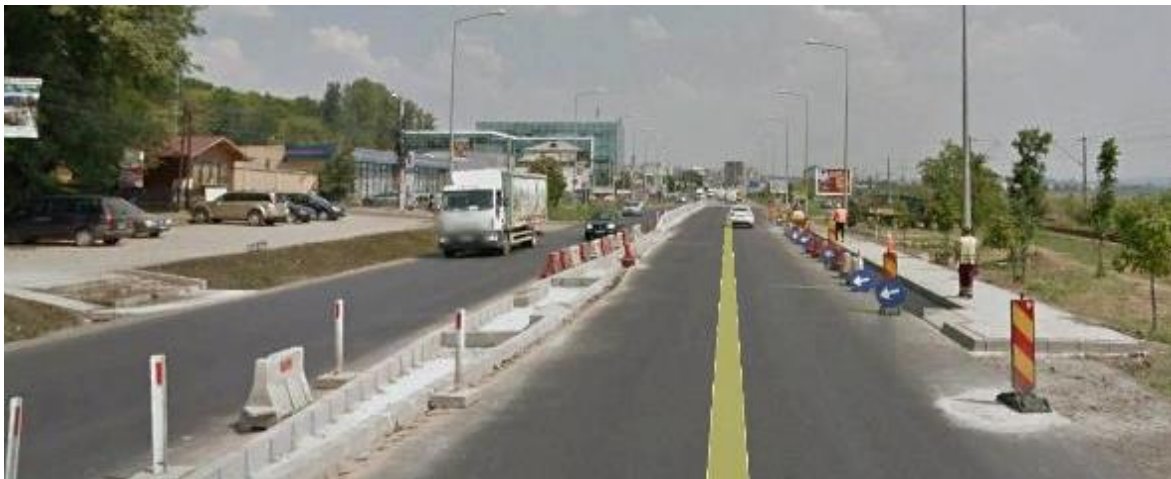
Figure 6.110 – During the intervention: construction site section 1, Iasi oriented view, details of the pedestrian refuge island
