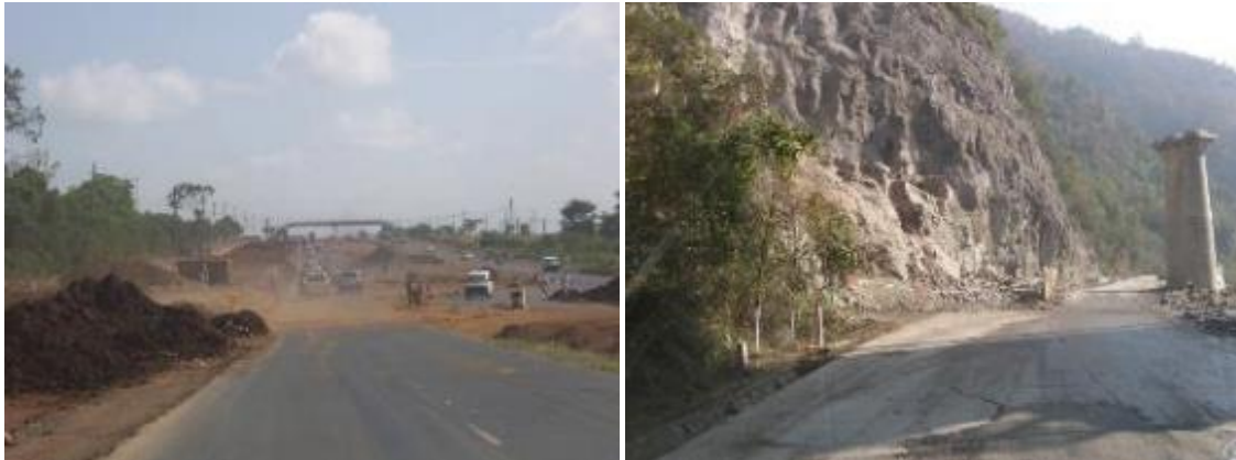
Figure 5.1 – typical examples of inadequate work zone arrangements
