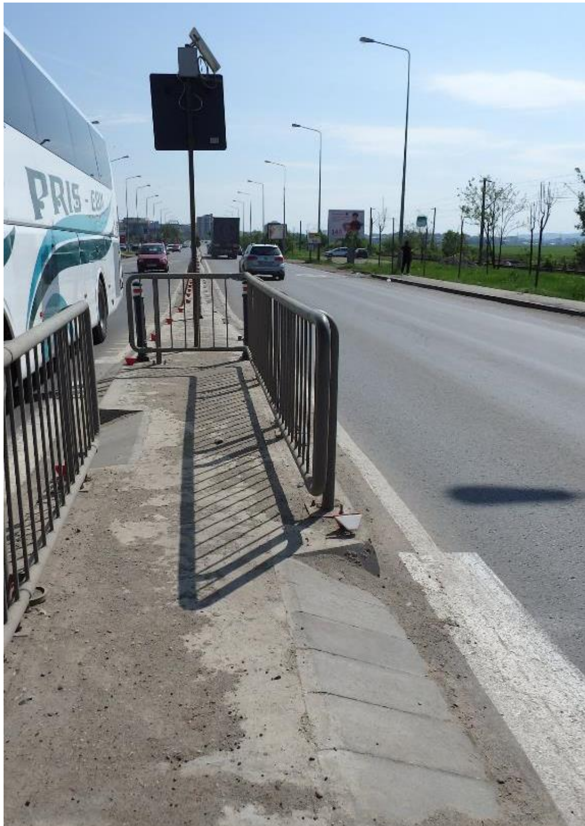
Figure 6.117 – After the intervention: road section 1, lasi oriented view, details of the pedestrian refuge island
